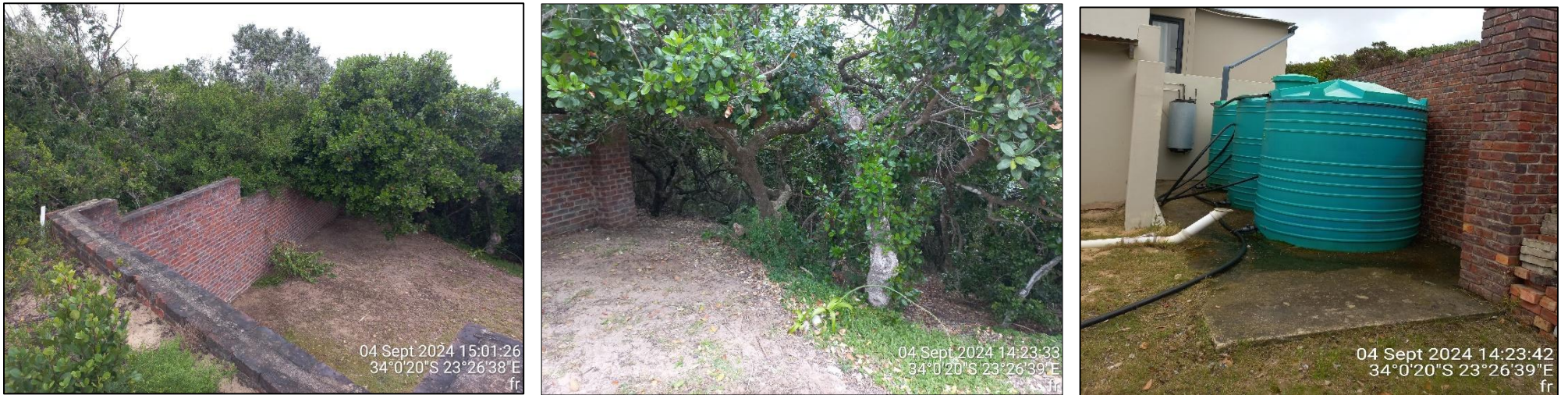
Figure 15: North-eastern corner, retaining wall of house platform. Note large Milkwood & tanks to be removed.
