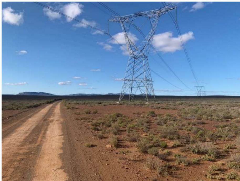
Figure 23. Image showing nature of the corridor to be traversed by the proposed electrical powerline serving the Kappa substation and existing powerlines proximal to the servitude in the Farm Die Brak.
