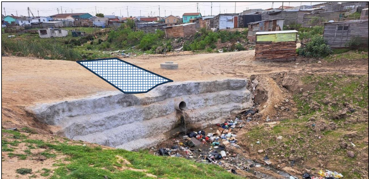
Figure 20: Proposed Reno mattress above the gabion wall to prevent erosion caused by blocked stormwater pipelines causing water to flow over the face of the gabion wall (Confluent Environmental, 2024).
