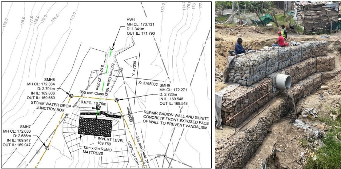
Figure 4. Diagram (left) showing plan view of the proposed reno mattress below the sewer line crossing supported by gabions. In addition, the location of a formalised stormwater headwall is proposed upstream (green dotted line). Inset photo shows emergency work undertaken to restore the sewer line crossing with potential for undercutting due to water falling at the toe of the gabions.
