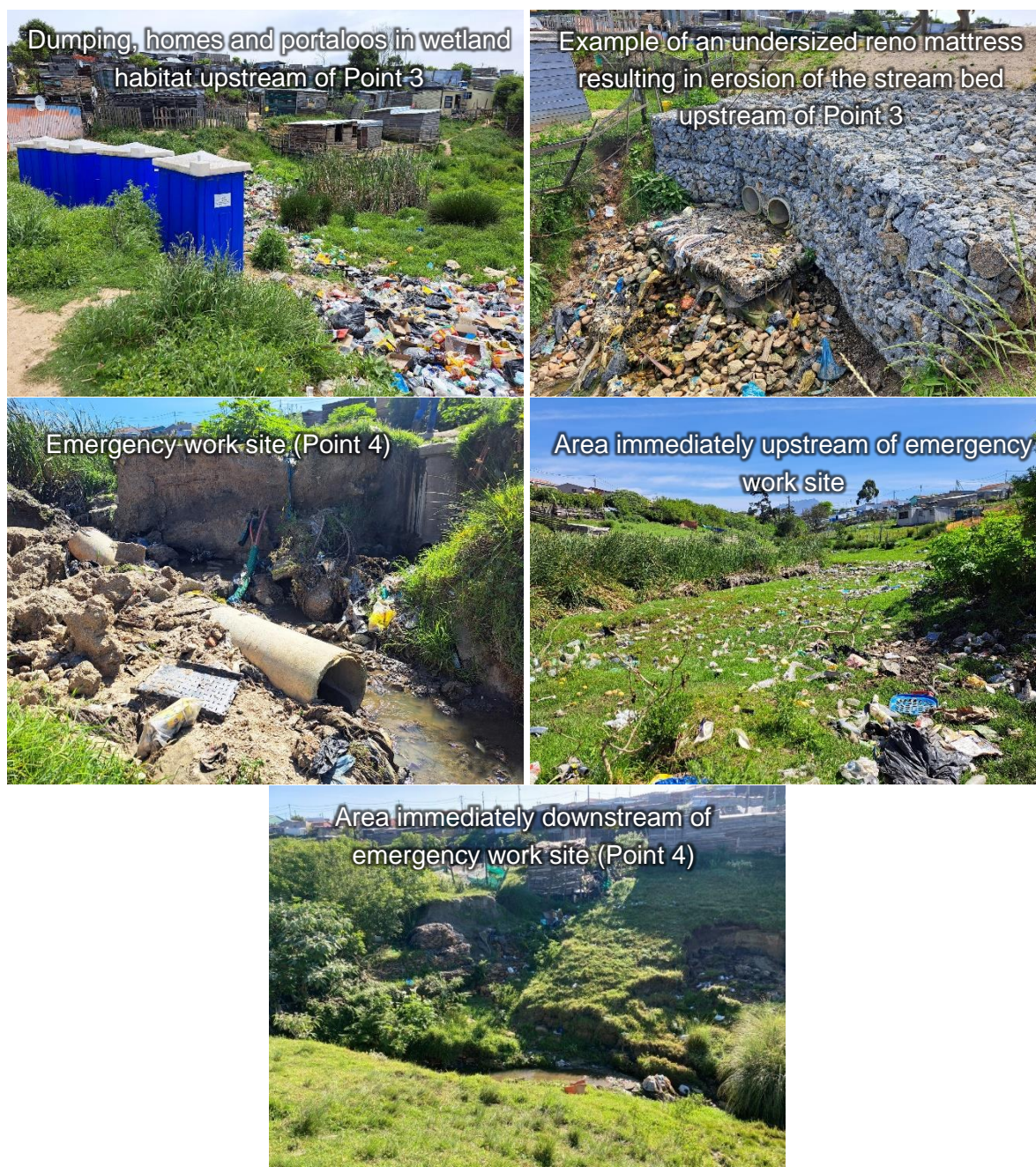
Figure 13. Photos of various site aspects taken during the site visit on 1 November 2023.
