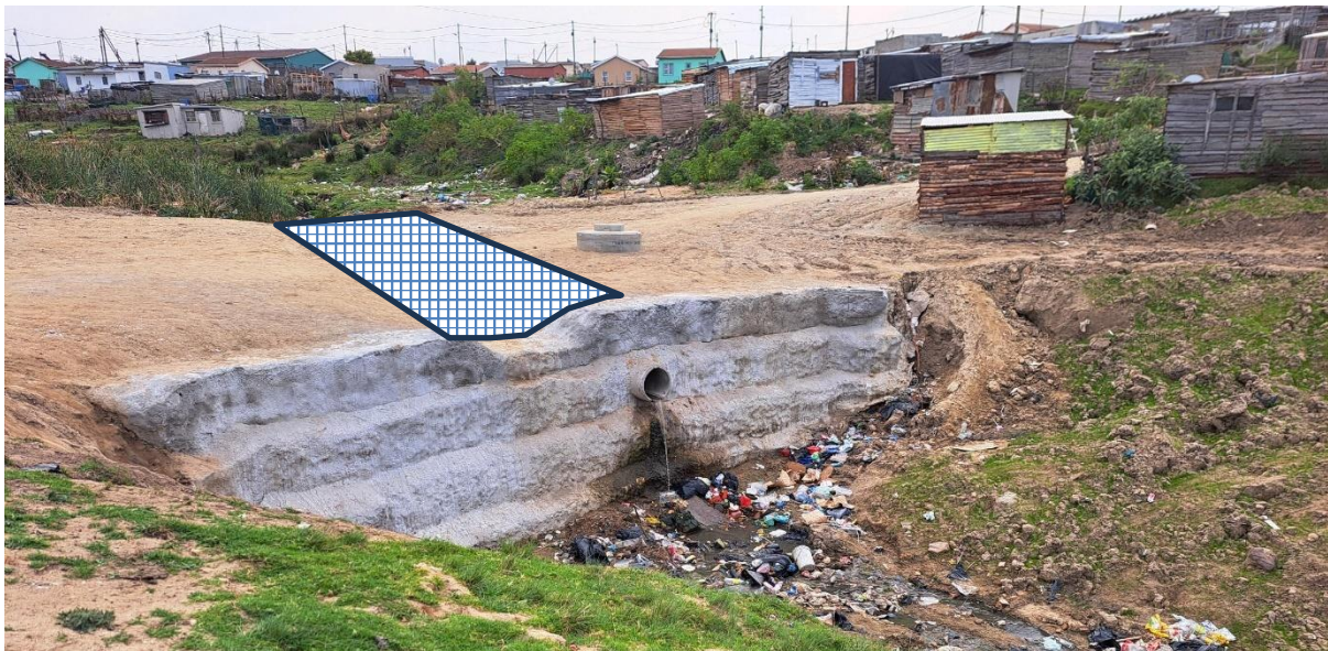
Figure 6. Photo taken of the almost completed emergency repairs indicating the need for a reno mattress below the piped outlet, and the proposed emergency overflow above the pipe where reno mattress protection is also recommended.
