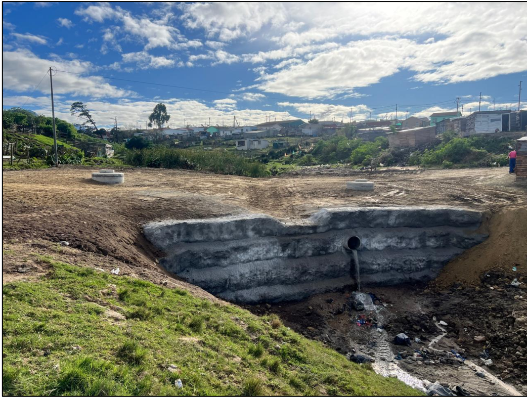
Figure 19: Newly constructed gabion wall. Reno mattresses proposed at the foot of the gabion wall to prevent erosion from plunging water in the stream bed. Reno mattress proposed above the gabion wall to prevent erosion caused by blocked stormwater pipelines causing water to flow over the face of the gabion wall.
