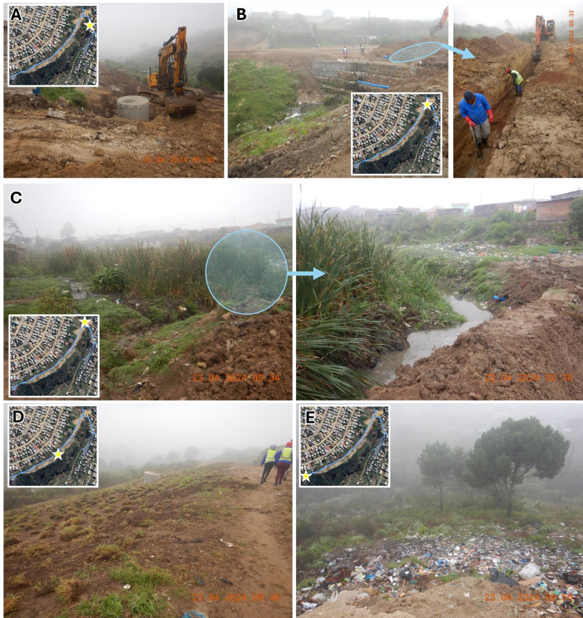
Figure 8: Images of the area where emergency repairs to the sewer line are taking place.
