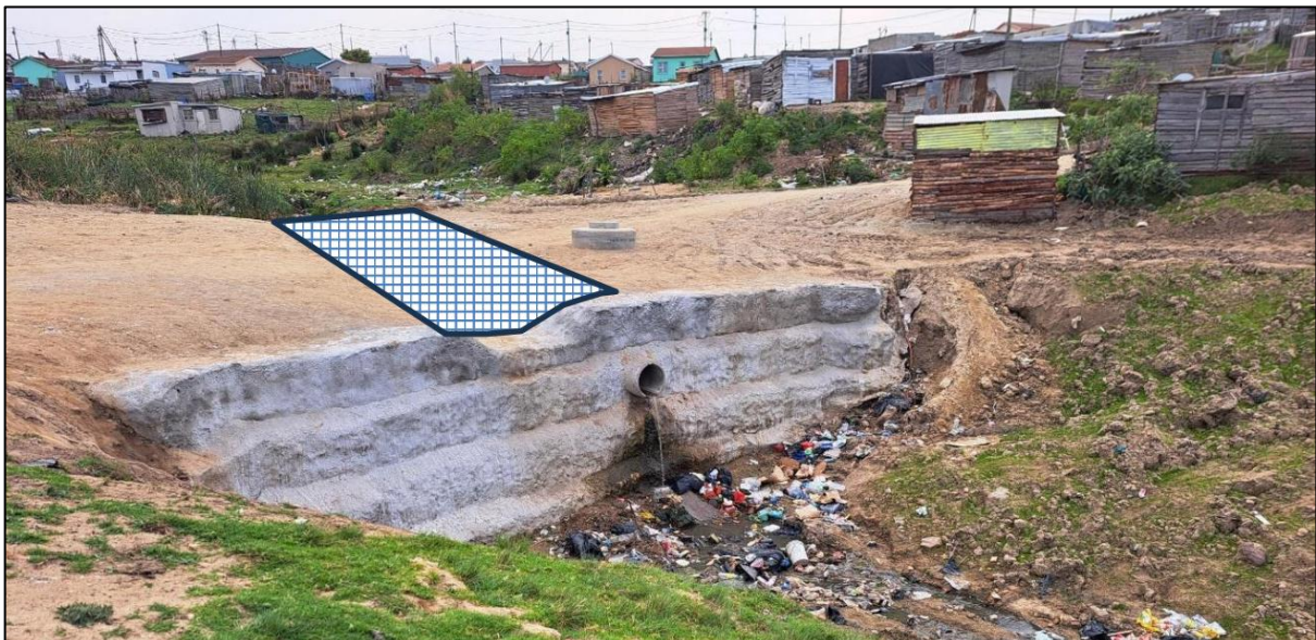
Figure 8: Proposed Reno mattress above the gabion wall to prevent erosion caused by blocked stormwater pipelines causing water to flow over the face of the gabion wall (Confluent Environmental, 2024).
