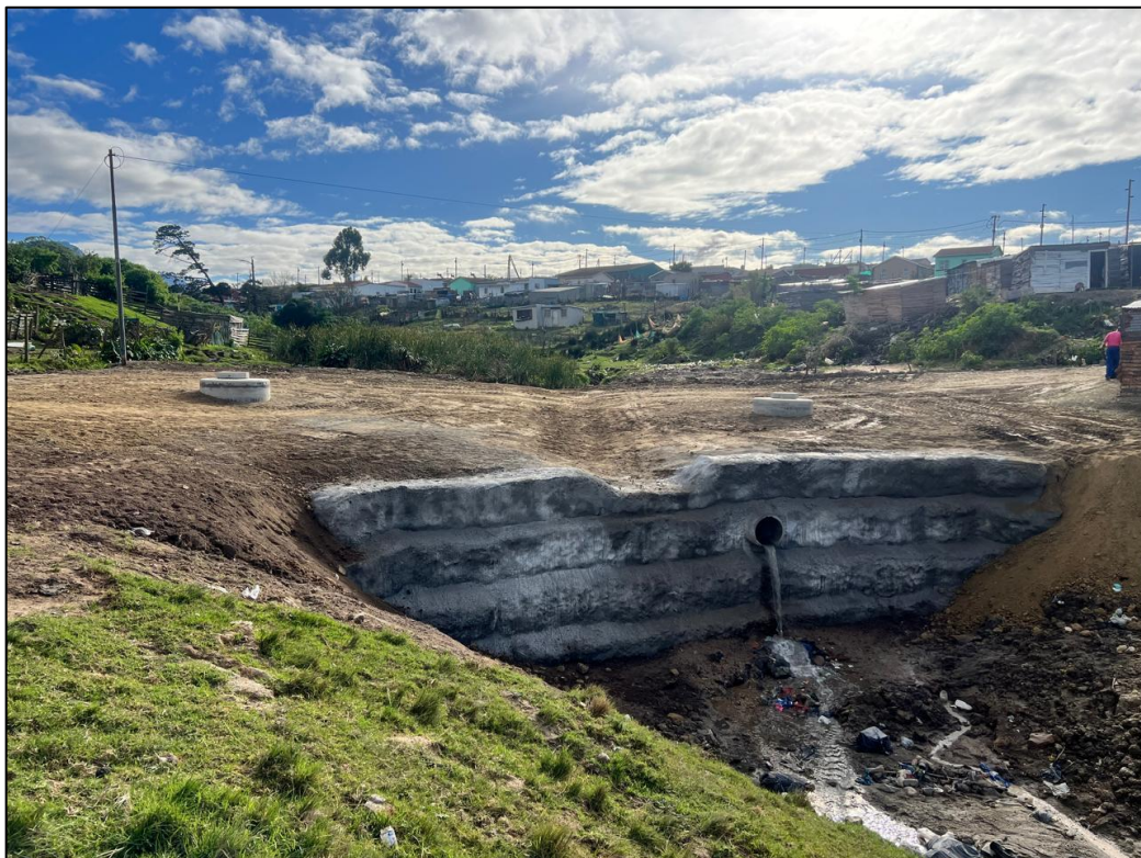
Figure 7: Newly constructed gabion wall. Reno mattresses proposed at the foot of the gabion wall to prevent erosion from plunging water in the stream bed. Reno mattress proposed above the gabion wall to prevent erosion caused by blocked stormwater pipelines causing water to flow over the face of the gabion wall.
