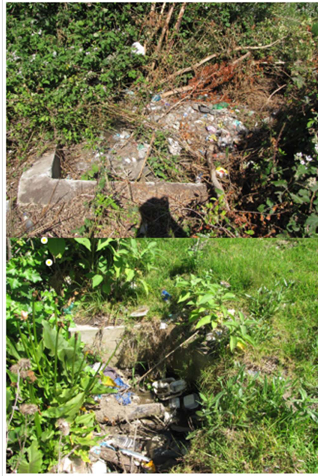
Figure 10. Litter and dense vegetation found at culverts across the road from the site. The poor quality of this water is a health risk for animals who use water in the landscape for their life functions.
