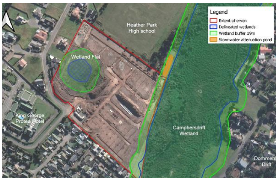
Figure 2: Study site under construction with overlay of wetland areas identified by specialists (Confluent Consulting, 2022).
