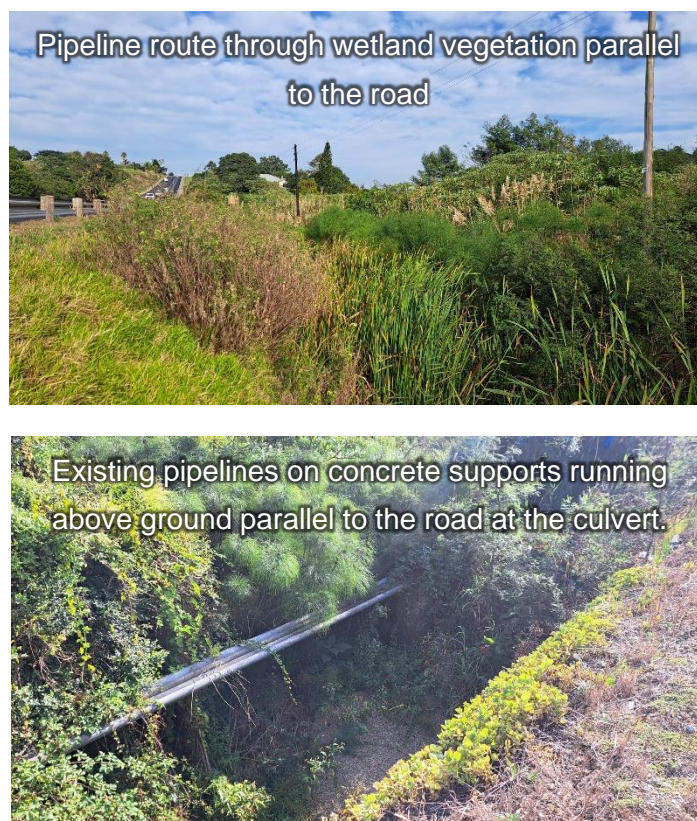
Figure 9. Wetland at crossing point B showing typical vegetation (top) and the existing pipelines opposite the culvert beneath the road (below).
