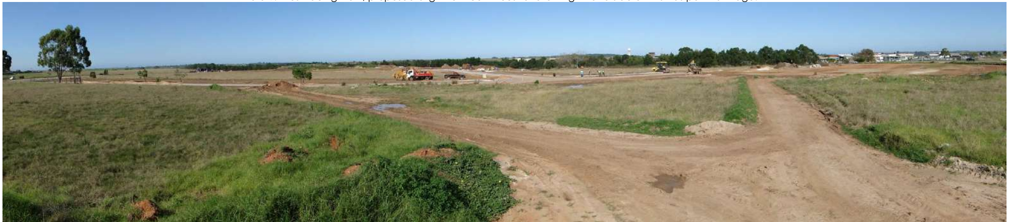
Photo 10: Southwest facing view across construction site directly opposite George Airport (visible in distance).
