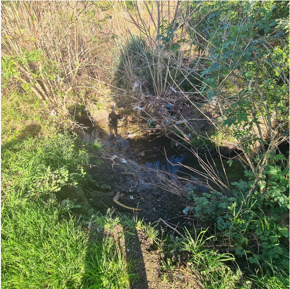
Figure 6: Degraded watercourse full of rubble.
