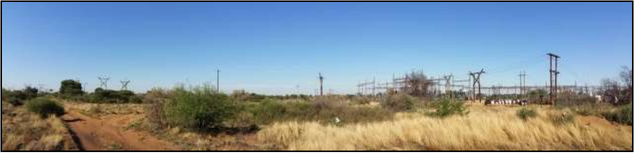
Figure 10: The Hotazel substation on the western edge of the town.
