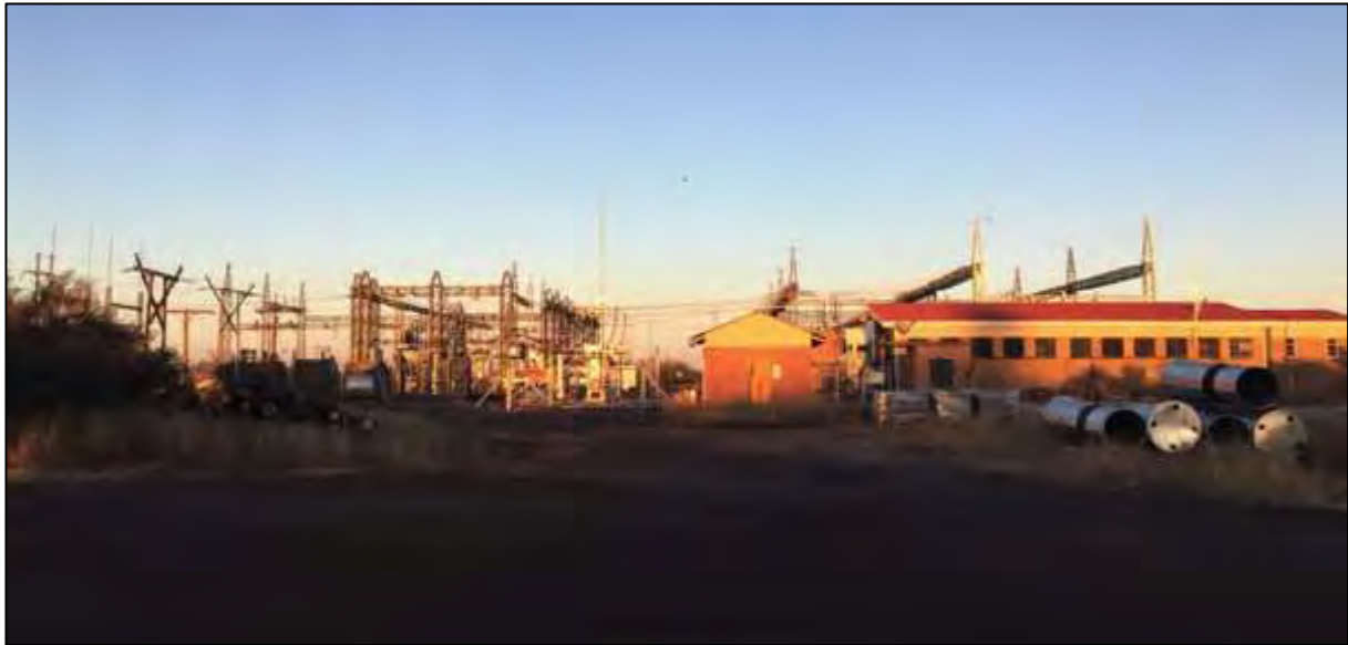
Figure 24: View west from Photo 6 of the existing Hotazel Substation to which the proposed power line would be routed.
