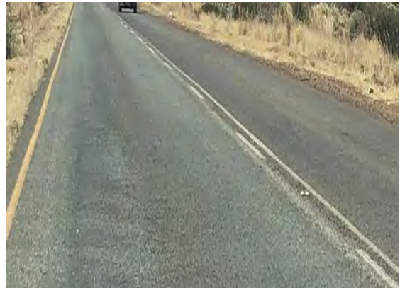
Photograph 3.2: Road markings on R31
