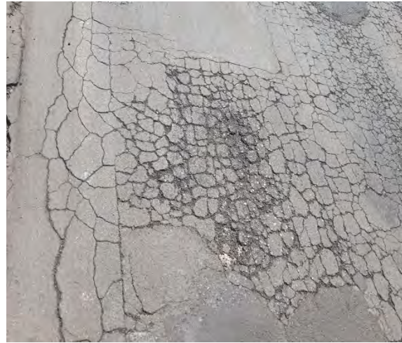
Photograph 3.4: Crocodile cracks in the pavement
