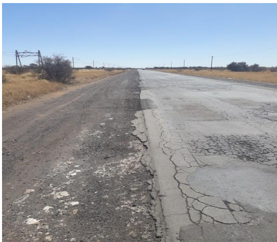
Photograph 3.5: non-existing road edge
