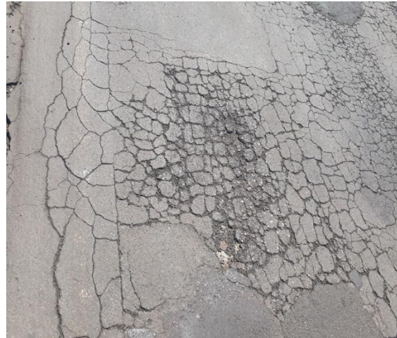
Photograph 3.4: Crocodile cracks in the pavement
