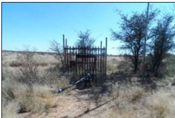
Borehole and pump OBS 05
