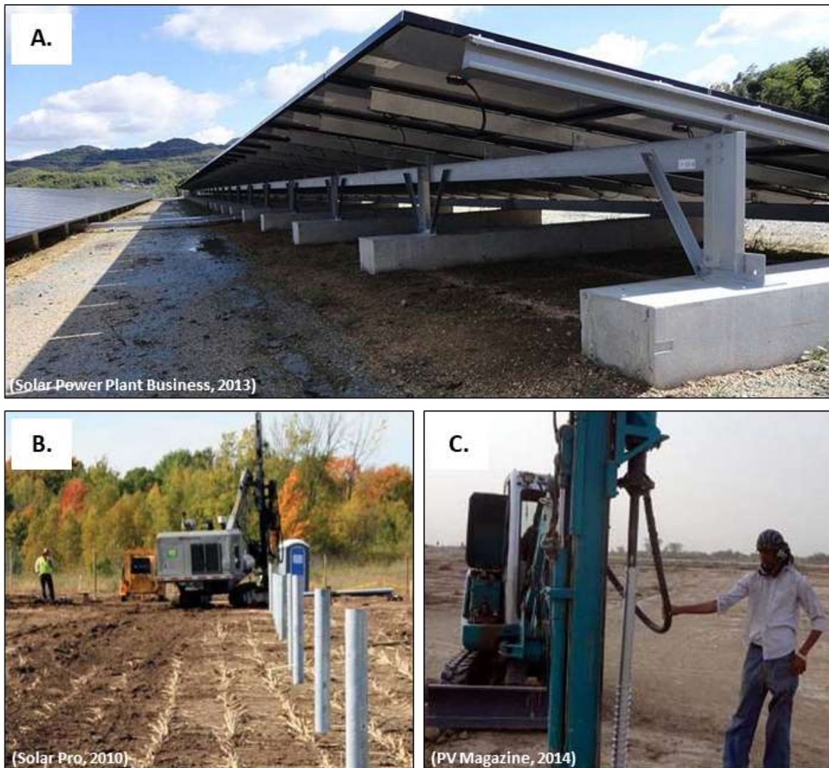
Figure 3: Mounting Structures. A) Cast Concrete Foundation. B) Driven/ Rammed Steel Pile. C) Ground / Earth Screw.
