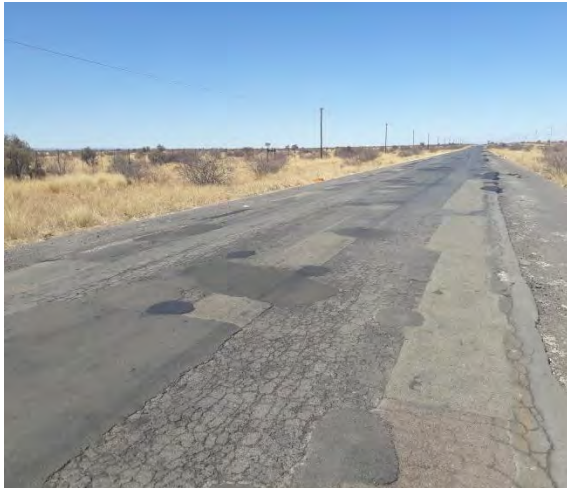
Photograph 3.3: Patching along the route
