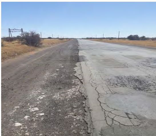
Photograph 3.5: non-existing road edge
