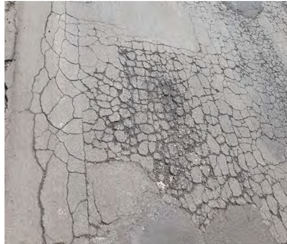
Photograph 3.4: Crocodile cracks in the pavement
