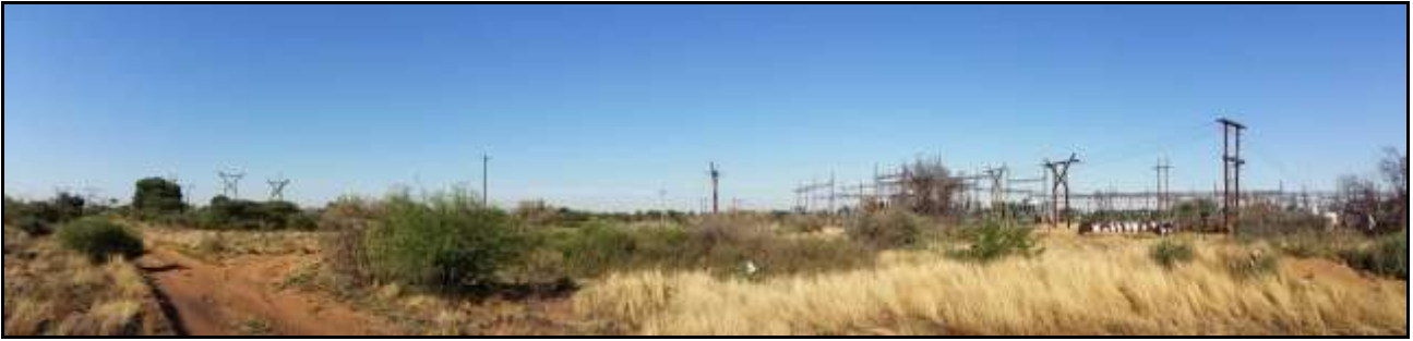
Figure 9: The Eskom Hotazel substation on the western edge of the town.
