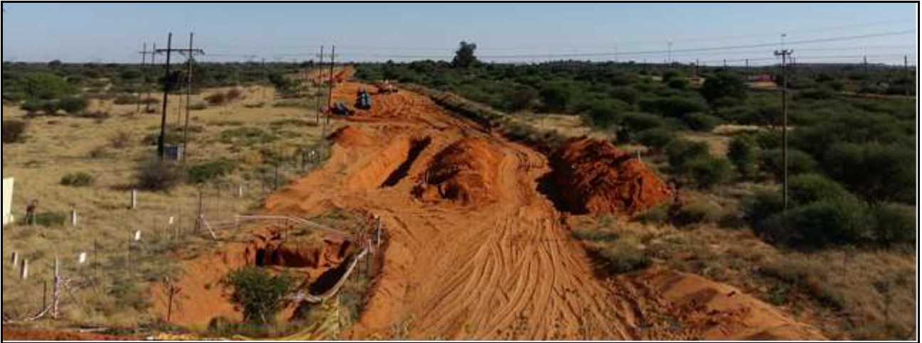
Figure 6: To the west of the railway line, large sections of the landscape on the Remaining Extent of farm York A 279 have been disturbed by the construction of an underground water pipeline which runs parallel to the railway line, and between the railway line and the R31. Note also the 66kV powerline which crosses the site from east to west.
