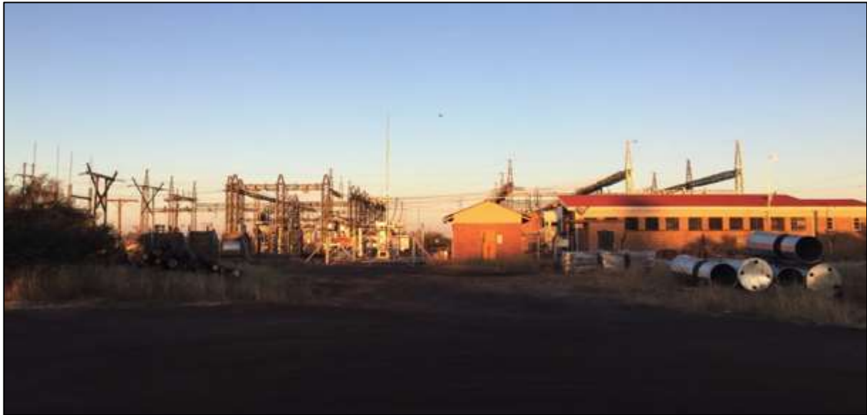
Figure 24: View west from Photo 6 of the existing Hotazel Substation to which the proposed power line would be routed.
