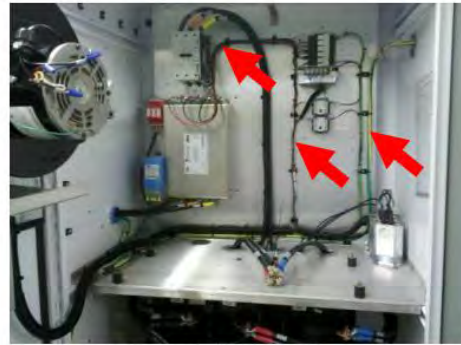
Controlled Wire Routing
