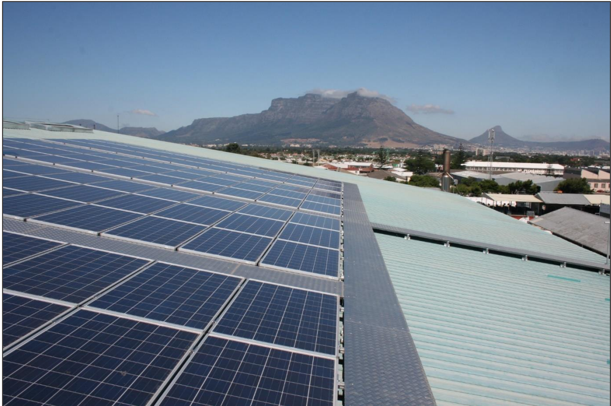
Figure 4.3: Solar Installations at the Cape Town International Airport in the Western Cape
