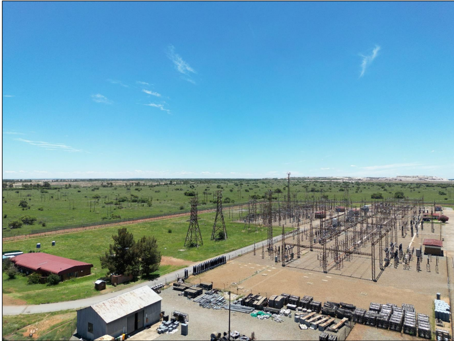
Figure 3.25: Aerial photo at Hermes Substation taken towards the north-west: AGL 30m
