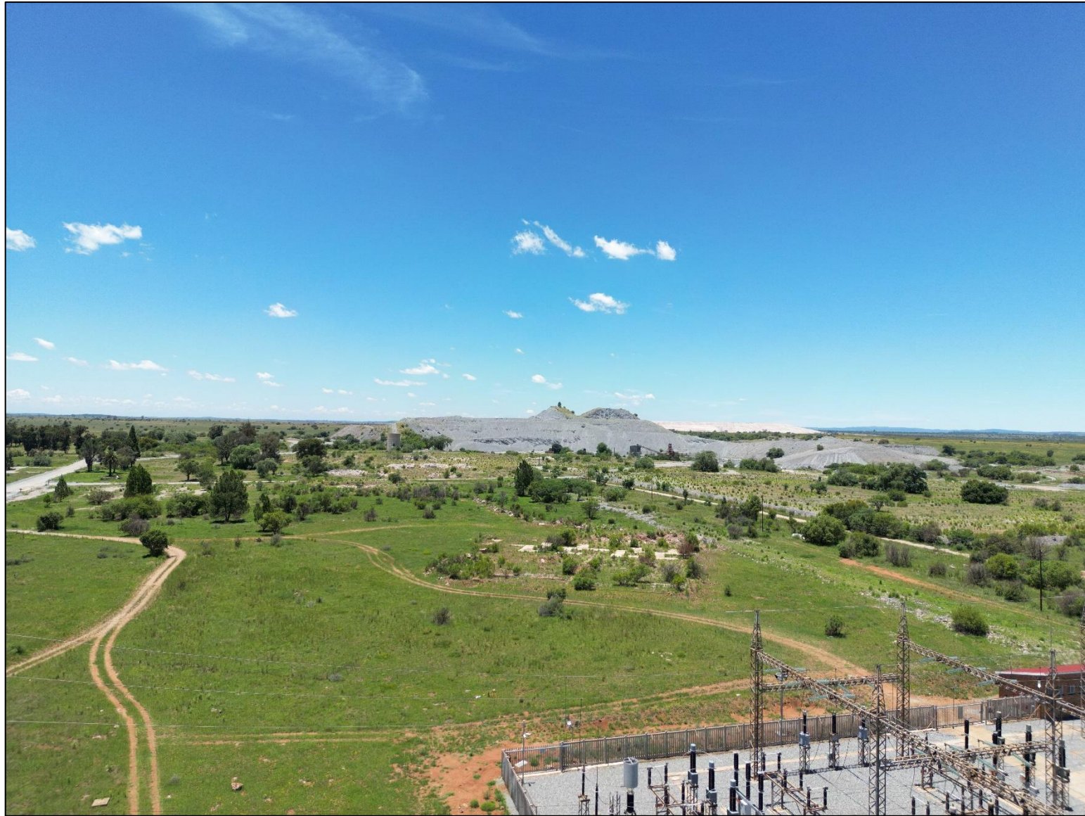
Figure 3.12: Aerial photo at Buffels East Substation taken towards the east: AGL 30m
