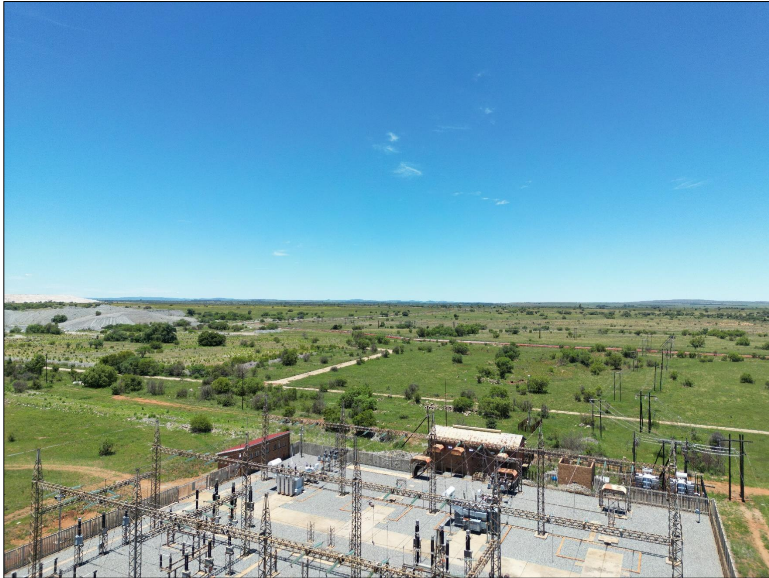
Figure 3.13: Aerial photo at Buffels East Substation taken towards the south-east: AGL 30m
