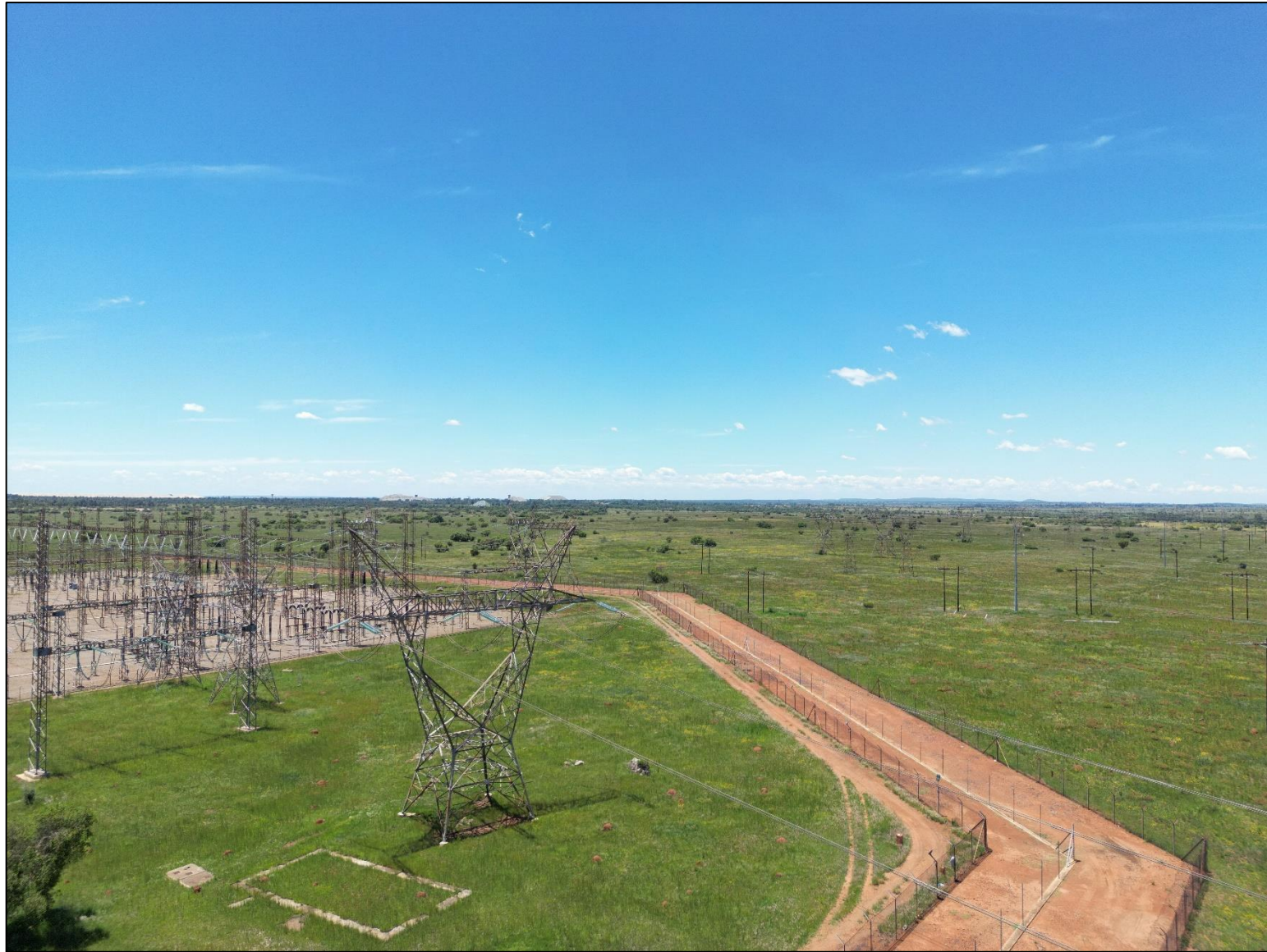
Figure 3.19: Aerial photo at Hermes Substation taken towards the north-east: AGL 30m
