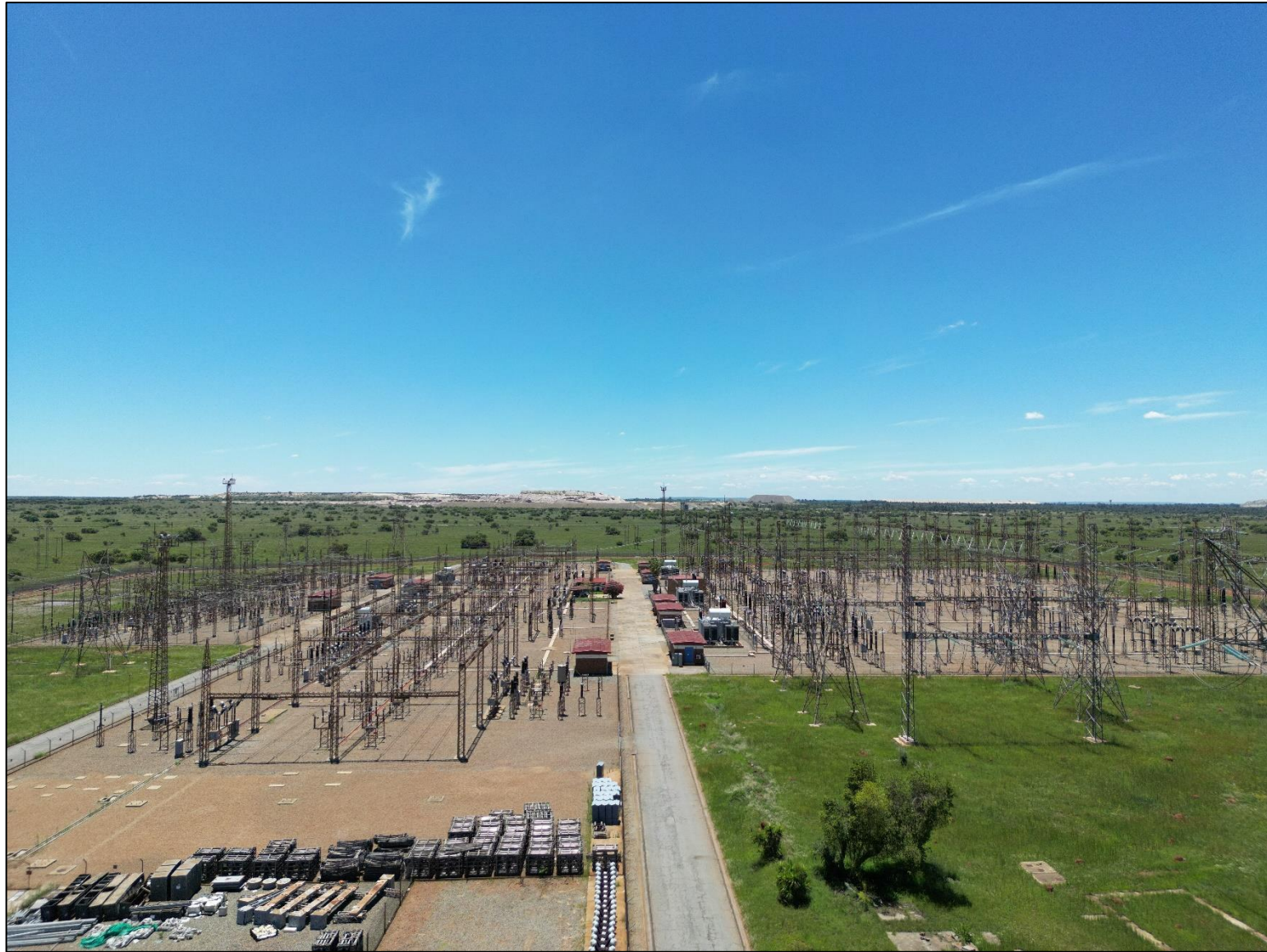
Figure 3.18: Aerial photo at Hermes Substation taken towards the north: AGL 30m
