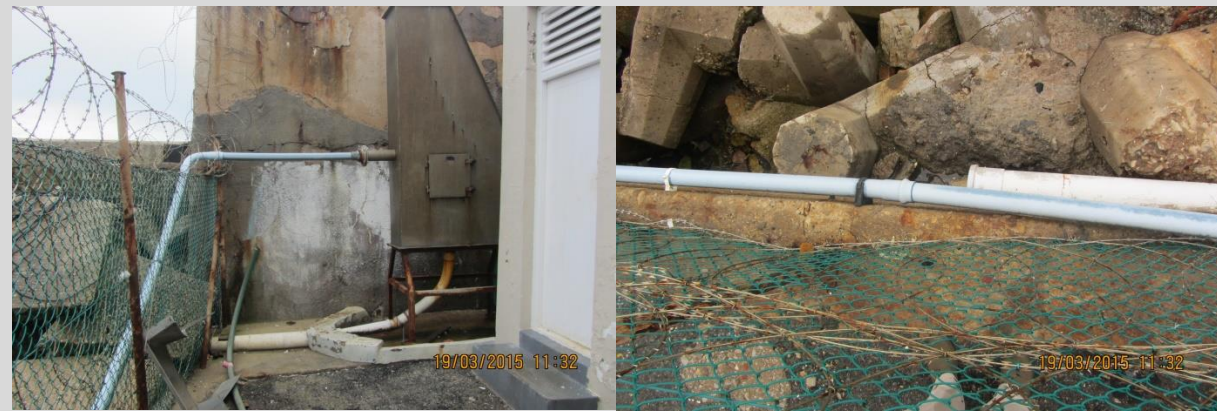
Photo 7: Sardine discharge enters the screen via the blue pipe and the discharge exists via the bottom white pipe
