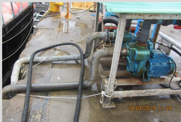
Photo 5: Abstraction of sea water takes place immediately adjacent to the quay
