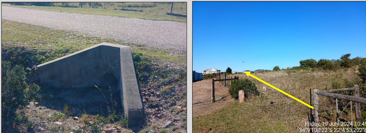
Figure 12: Left Photograph: Existing culvert underneath Klipheuwel road. Right Photograph: Proposed route for 600mm stormwater pipeline on 208/220.
