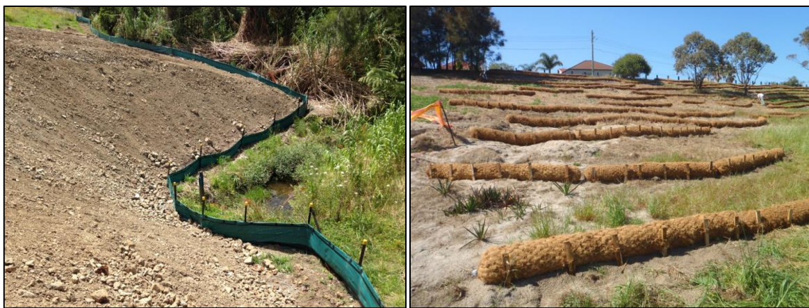
Figure 7: Examples of silt fences (left) and coir logs (right) used to trap sediment mobilised from steep slopes.
