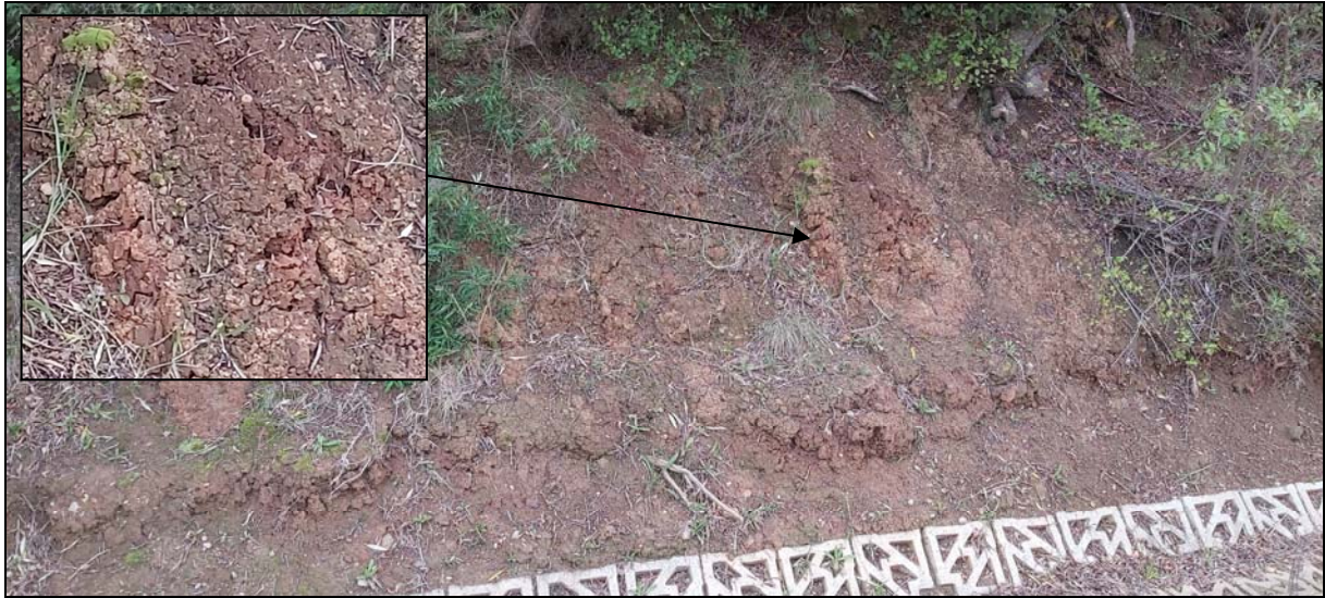
Figure 6: Reddish orange clayey soil profile exposed in road cutting along southern boundary of the site (inset: shattered clay structure)
