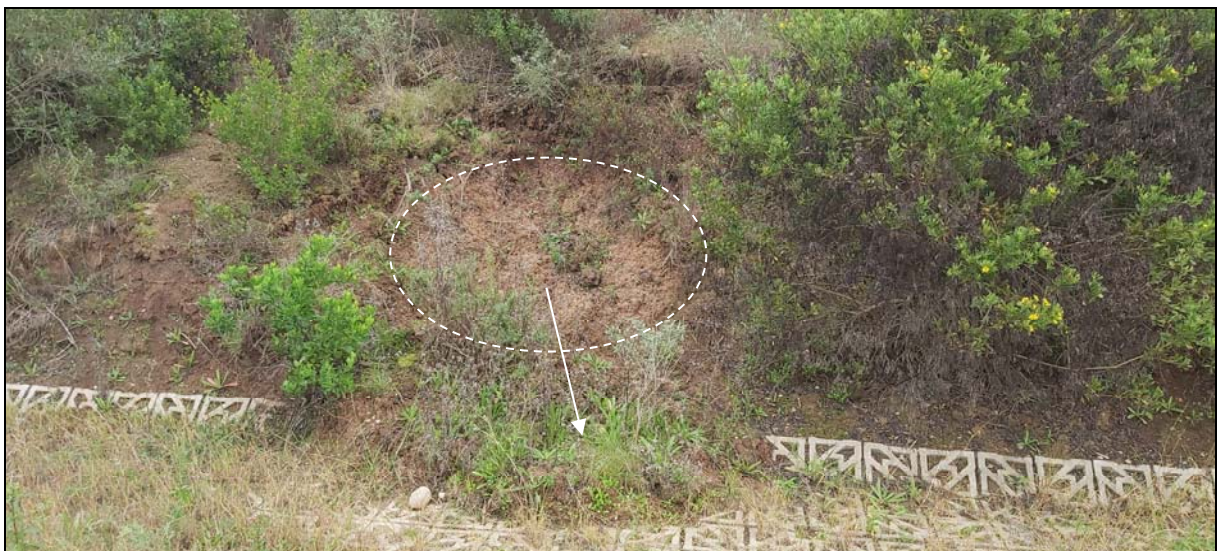
Figure 7: Small soil slip on the road cutting along the southern boundary
