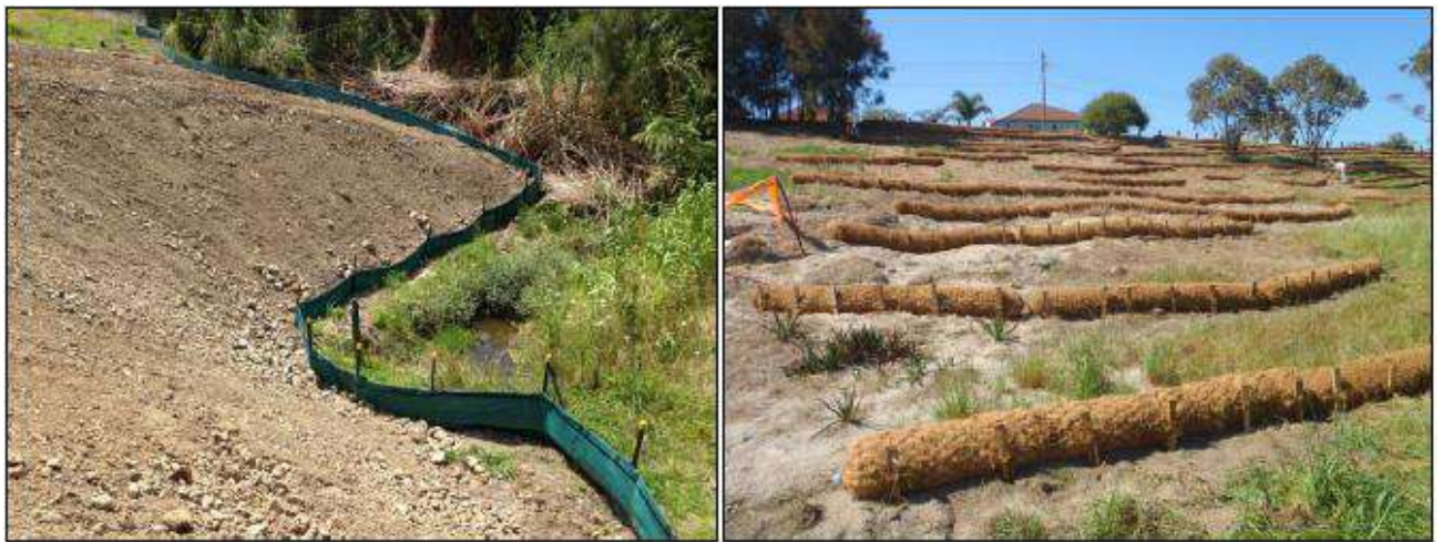
Figure 5: Examples of silt fences (left) and coir logs (right) used to trap sediment mobilised from steep slopes.
