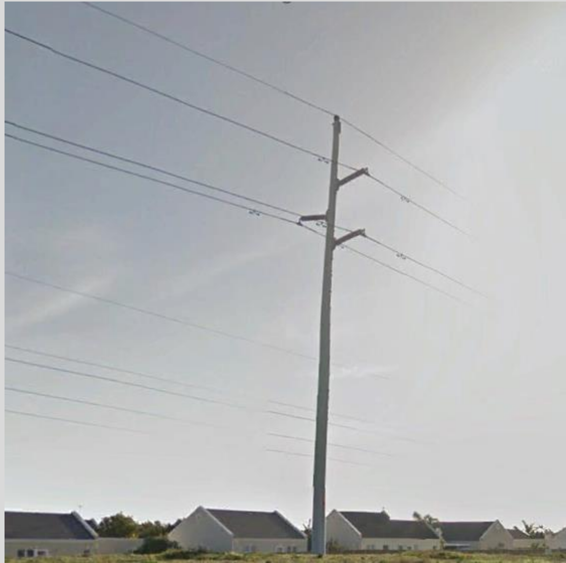
Figure 12: Photographic Example of 132Kv Monopole Pylon
