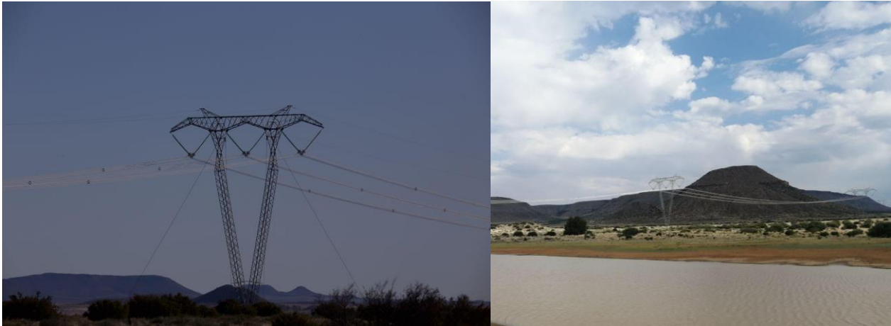
Figure 3-6: Artificial habitat created by electricity powerlines and pylons in or near the Kareekloof EGI study area.
