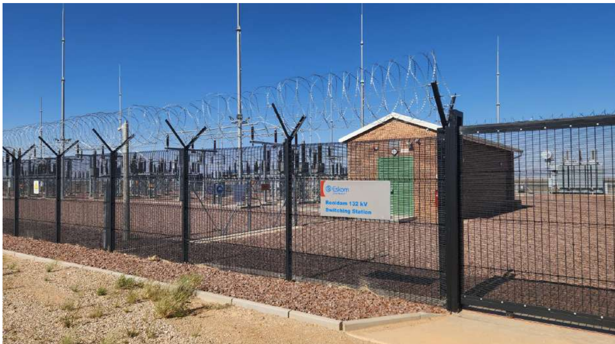
Figure 14: Example of typical substation with the Eskom Portion in the foreground and IPP Portion in the background (Photo: Cape EAPrac, 2024).
