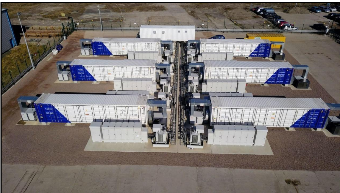
Photograph 1.2: Example of BESS located in storage containers
