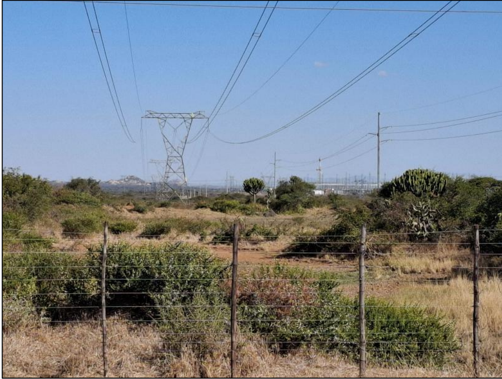
Photograph 3.8: Eskom transmission lines entering Tabor Substation
