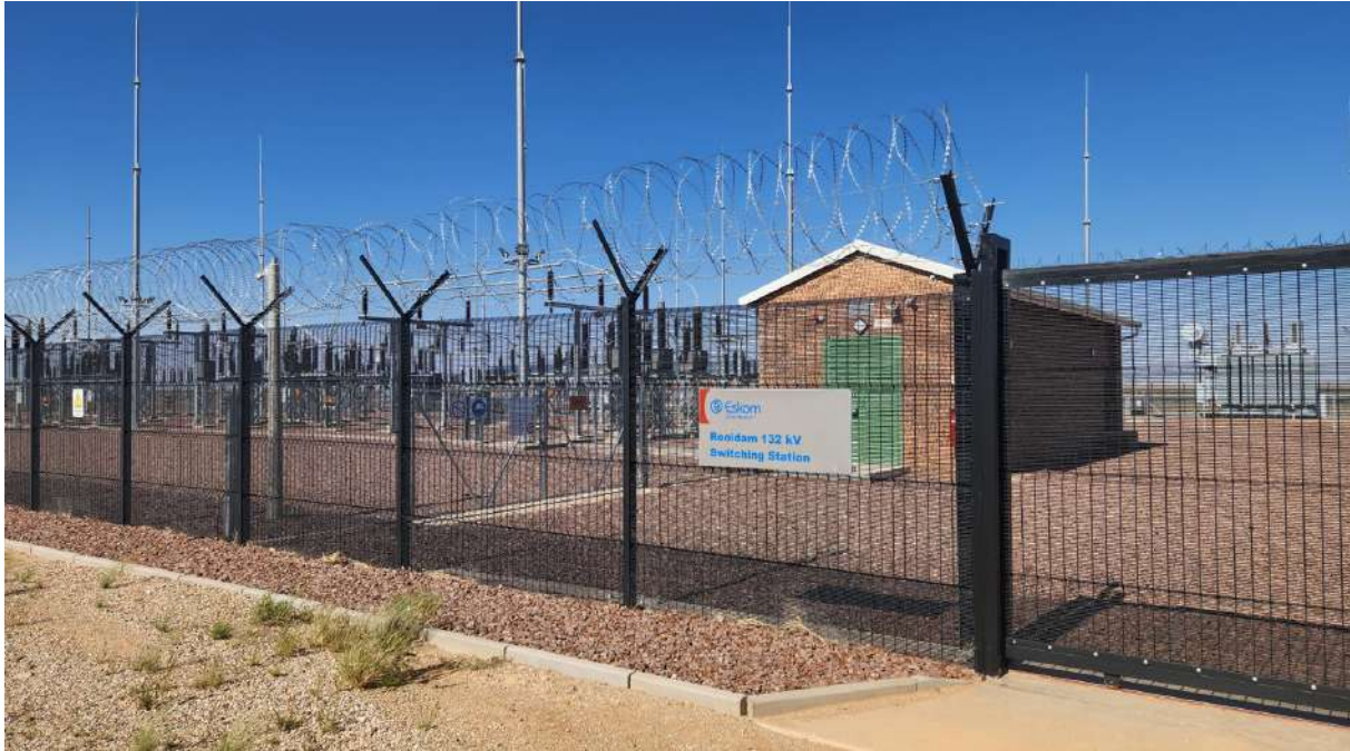
Figure 13: Example of typical substation with the Eskom Portion in the foreground and IPP Portion in the background (Photo: Cape EAPrac, 2024).
