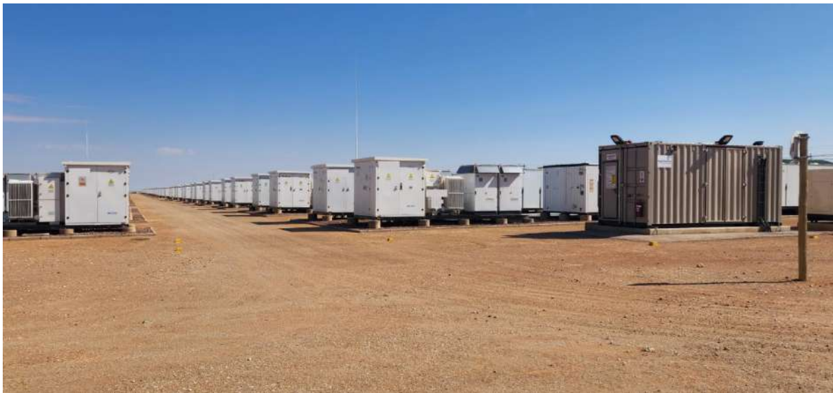
Figure 15: Example of typical newly constructed Solid State Lithium Ion BESS (Photo: Cape EAPrac, 2024).
