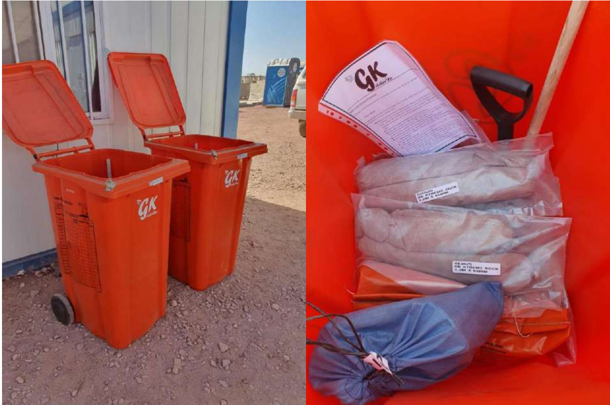
Figure 19: Hydrocarbon Spill Kits must be in place within the site camp, at each work area and in the field within 500m of any drilling or ramming activity.
