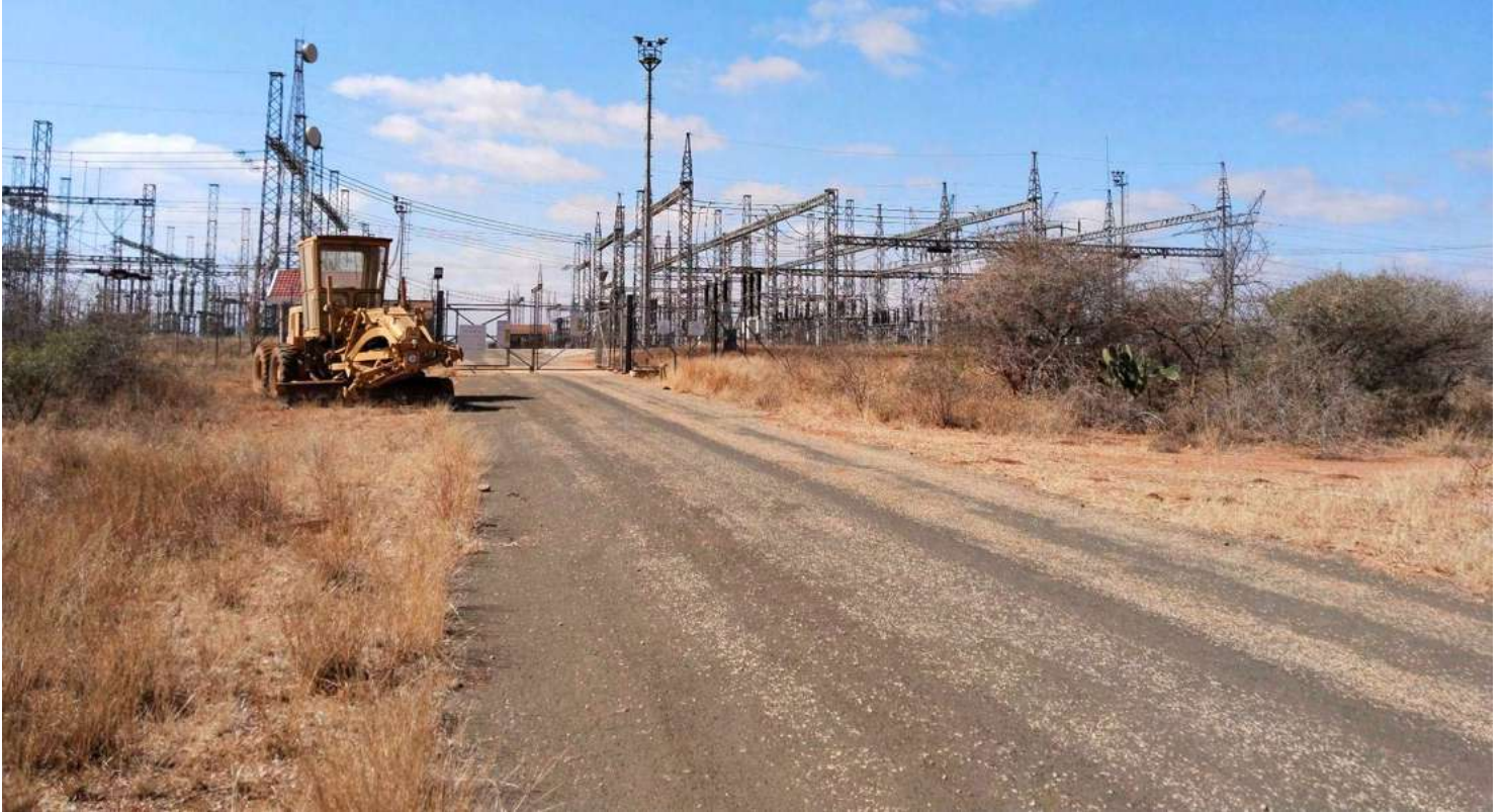
Figure 4.21: View of Tabor substation.
