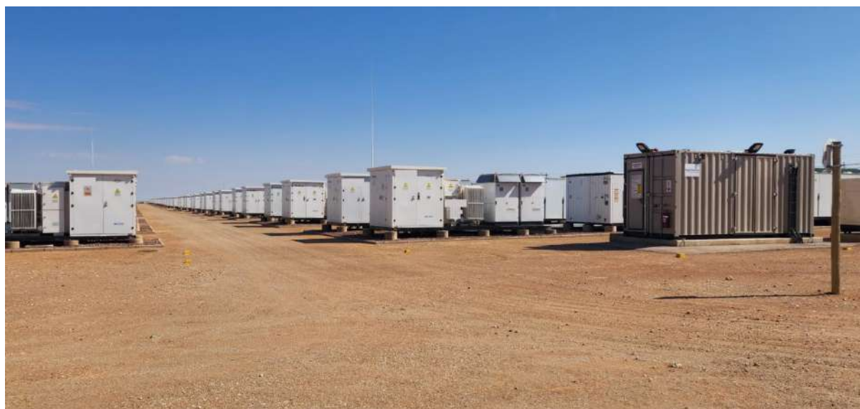
Figure 16: Example of typical newly constructed Solid State Lithium Ion BESS (Photo: Cape EAPrac, 2024).
