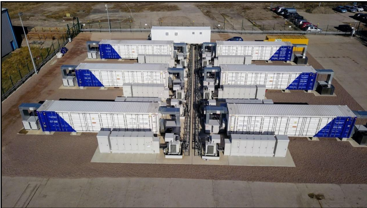
Photograph 1.2: Example of BESS located in storage containers
