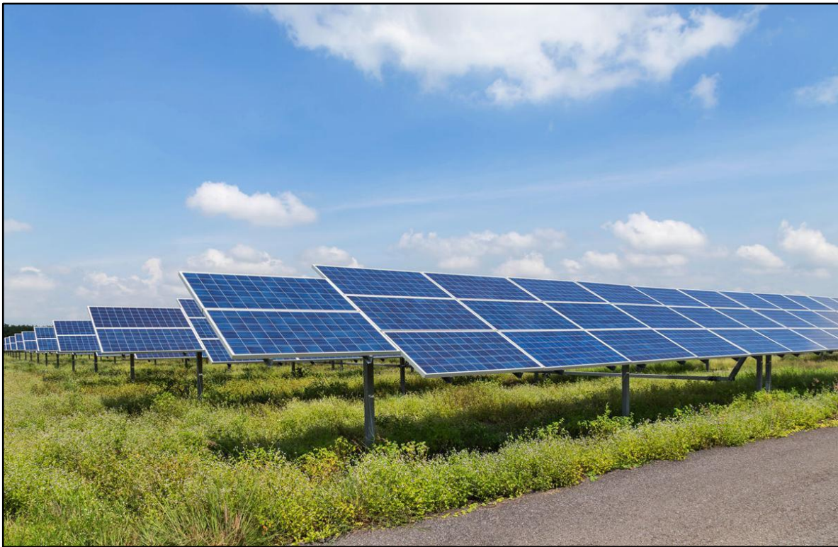
Photograph 1.1: Typical PV SEF facility
