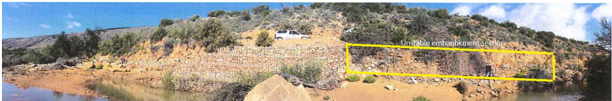
Figure 1: Vrede Goedehoop Road - Extend of Eroded embankment
