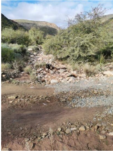
Figure 9: photo 28, a seasonal watercourse area intersecting the road. The road edge is strewn with boulders, cobbles, and sediment.
