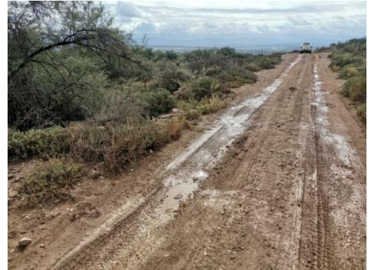
Figure 17: photo 59, muddy, saturated conditions. And standing water in depressions.
