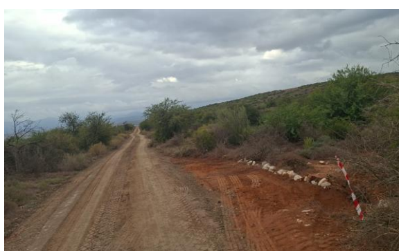
Figure 14: Example of temporary designated passing bay along narrow track to enable large construction vehicles to pass each other. Area must be clearly marked and rehabilitated once repair work is completed.
