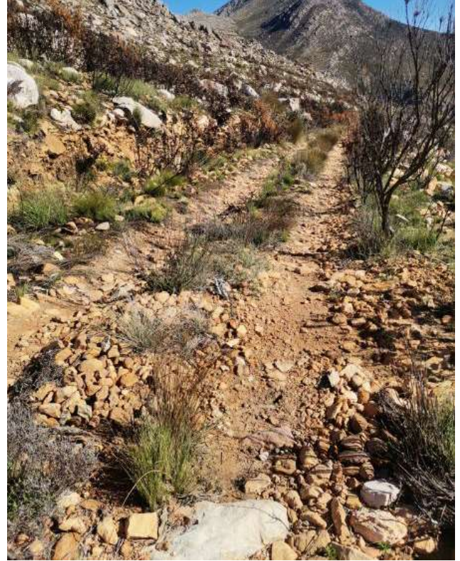
Figure 24: Photo 81, roadway eroded with exposed rocks, no adequate stormwater drainage.
