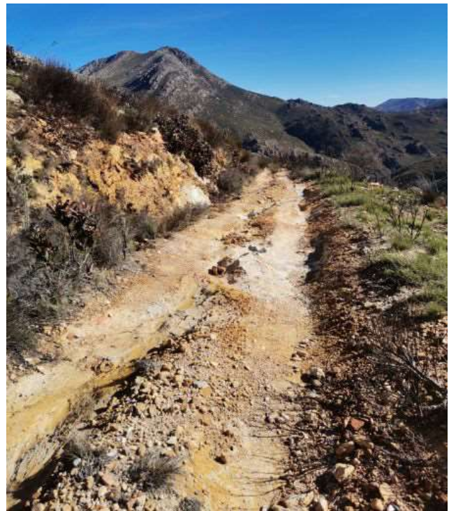
Figure 22: Photo 78, the road in average condition. Reshaping of humps required.
