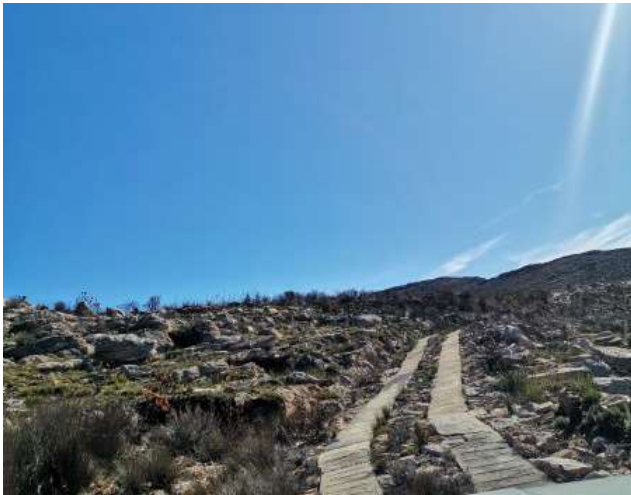
Figure 9: Photo 17, road in good condition. Concrete strips are still in good condition.
