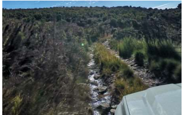
Figure 28: Photo 91, the road is in poor condition. Wheel tracks eroded, rocks exposed and water standing in wheel tracks.
