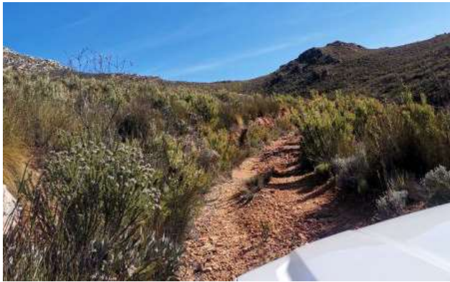
Figure 29: Photo 98, road in average condition. Reshaping of humps required.
