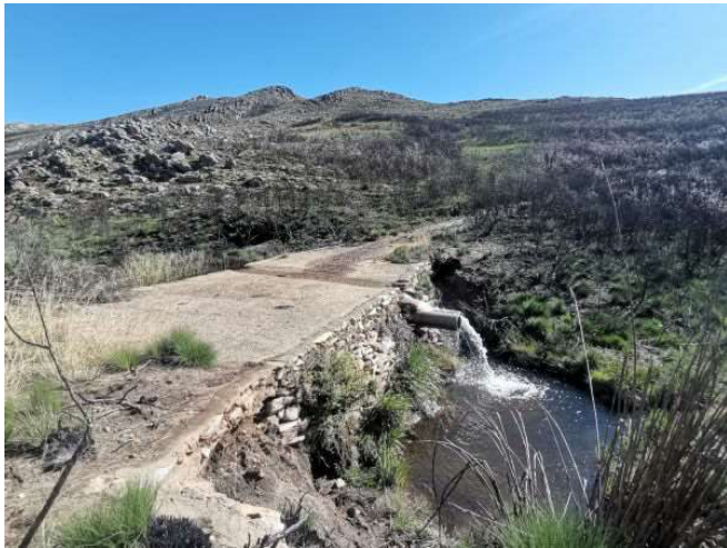
Figure 5: Photo 4, concrete slab bridge in good condition. No remedial action required at the bridge.
