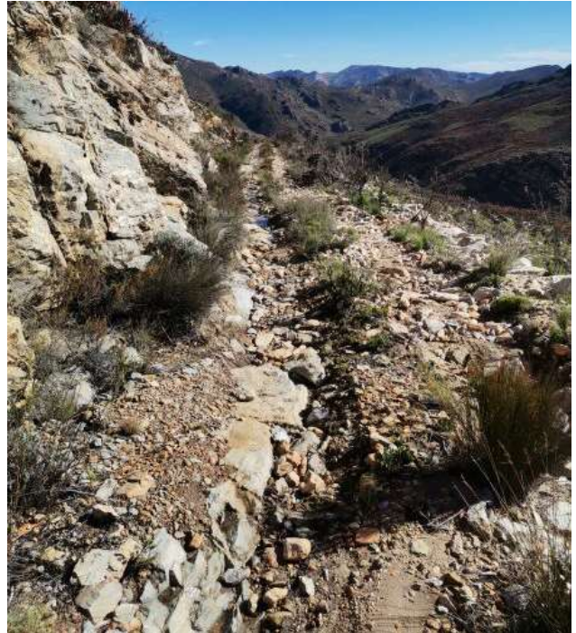
Figure 20: Photo 67, road in poor condition. All fines eroded. Large rocks exposed.
