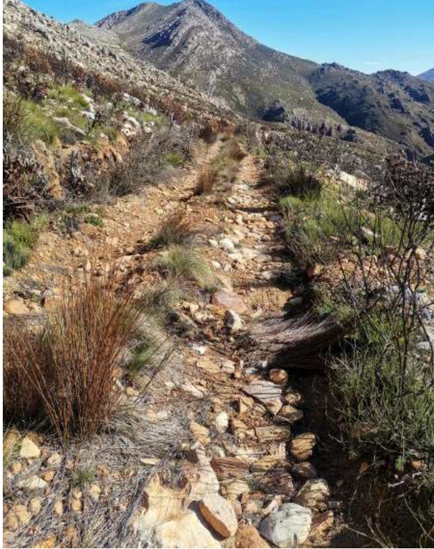
Figure 23: Photo 80, soil eroded, humps required to channel the water out of the road path.
