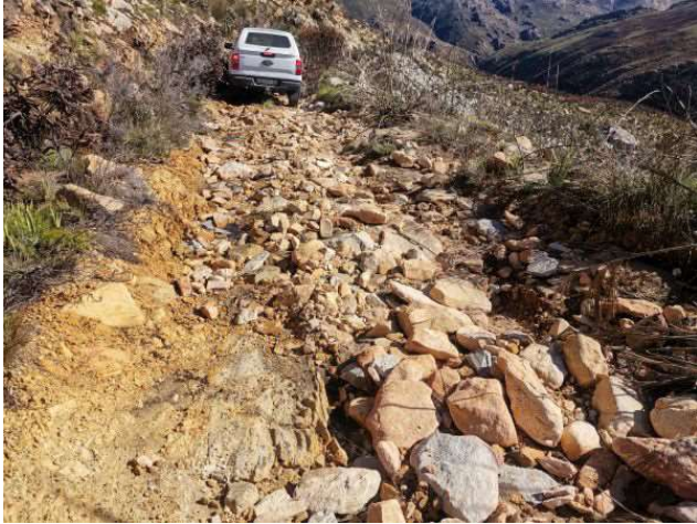
Figure 19: Photo 65, road is in critical condition. All fines eroded. Large rocks exposed.
