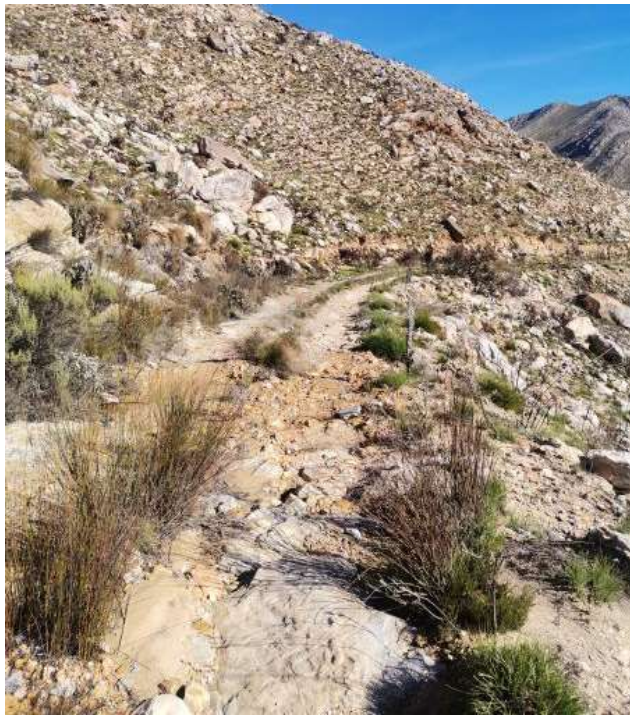
Figure 21: Photo 72, road path is in poor condition. Wheel tracks eroded.
