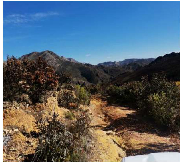
Figure 18: Photo 57, rock in poor condition. Evidence of stormwater running along road and soil washed away. Humps required to direct water away from road
