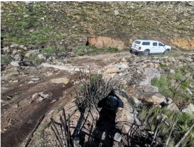
Figure 17: Photo 52, road is in poor condition. Eroded with large rocks exposed.
