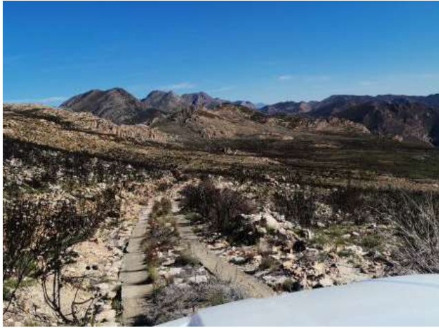
Figure 15: Photo 33, concrete strips in average condition. Cracking and some movement visible.
