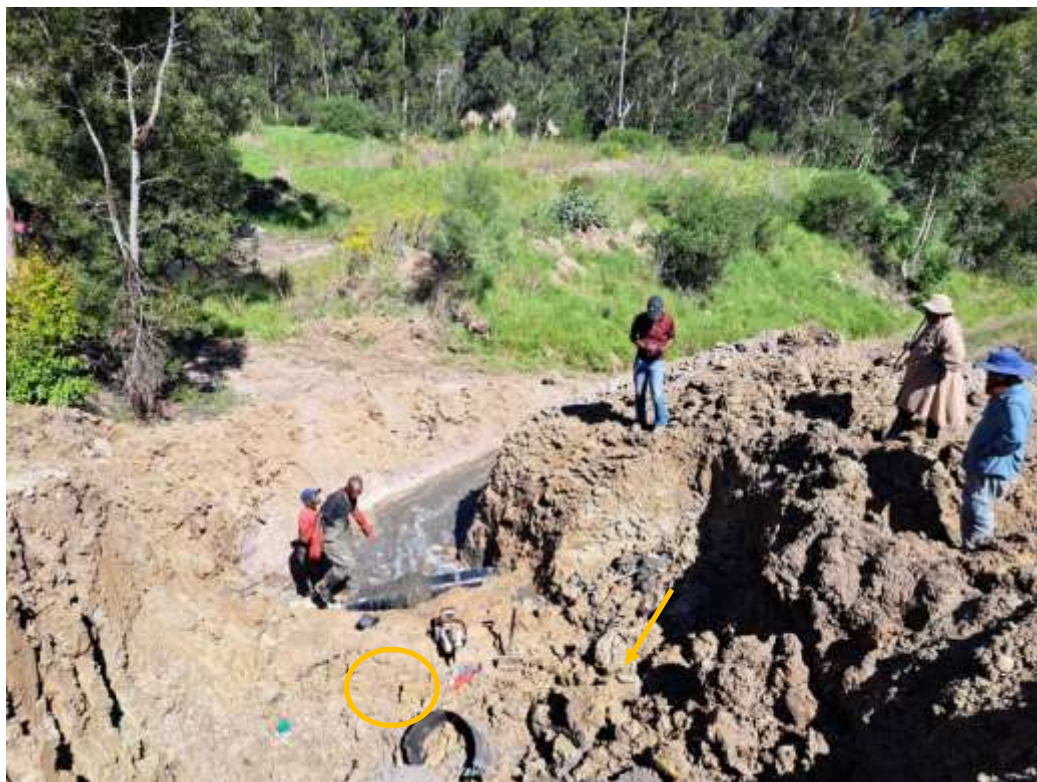
Figure 9. Photo taken on 31 March 2023 of a bulk sewerline that was opened to remove a blockage due to a walking crutch (arrow). Raw sewage and silt flowed straight downslope into the Bigai Wetland.
