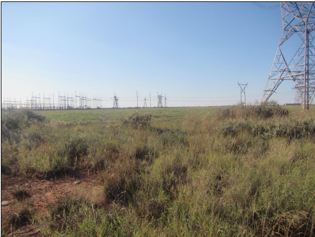
Figure 10: Looking north towards the Ferrum Substation.
