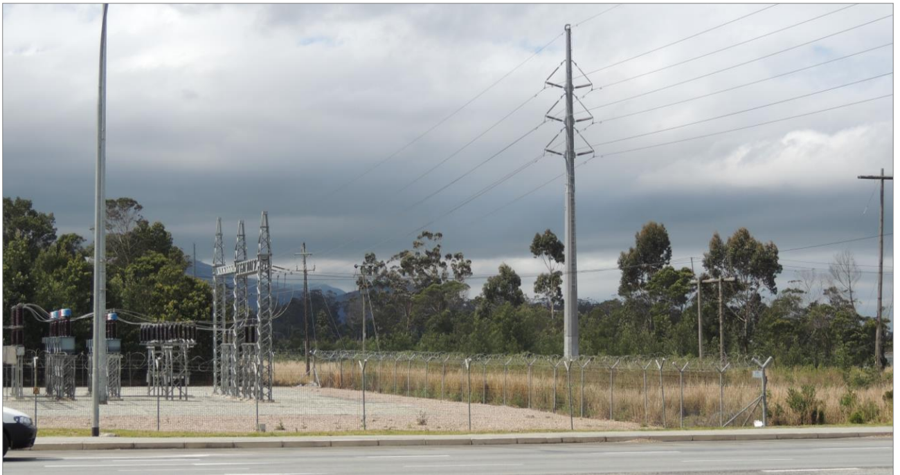
Figure 2: Example of monopole transmission lines link to a small substation (Source: VRMA)
