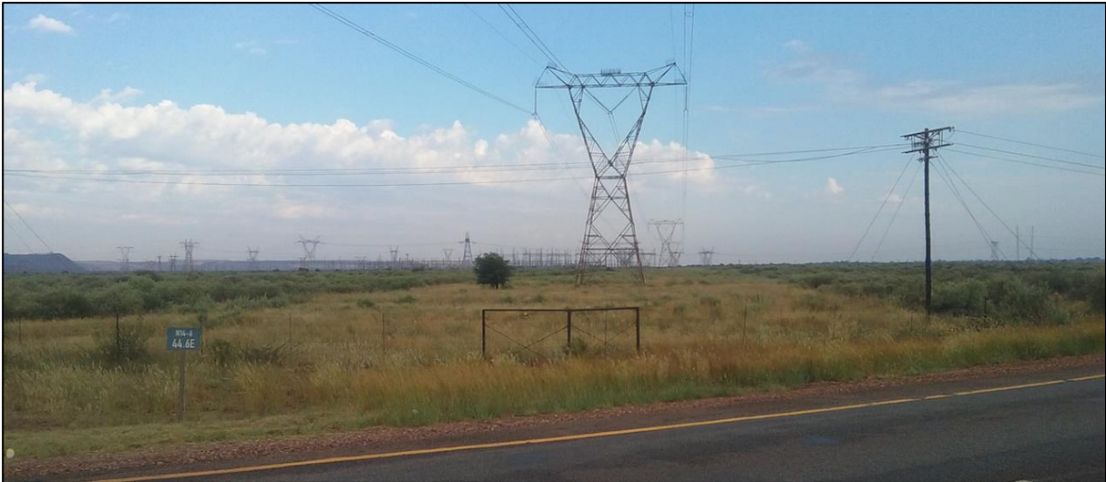
Figure 6: Photograph of the Ferrum Substation and 400kV powerlines leading to the substation (Source: D. Holder Cape EAPrac 2018).
