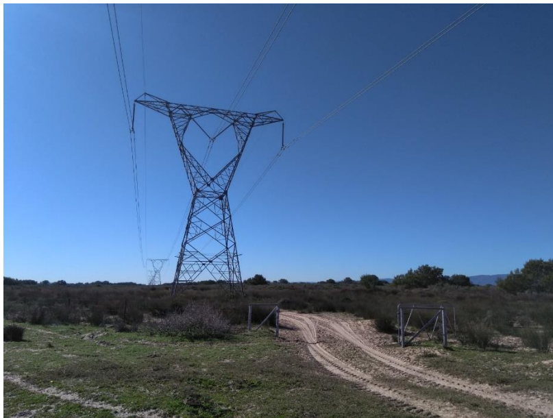
Figure 3: High voltage power line in the Project Site.
