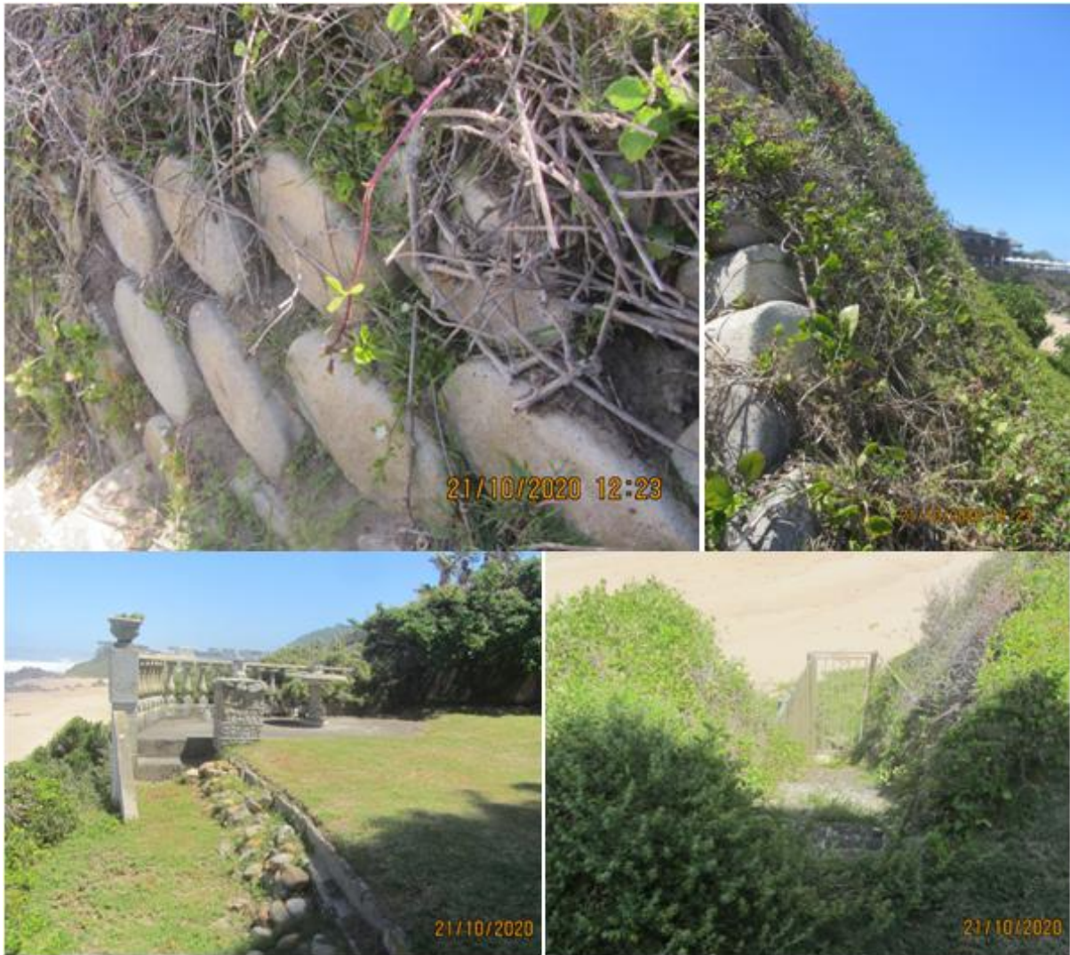
Figure 6: Photographs showing the interlocking concrete block retaining wall, stairway and upper concrete retaining wall / viewing deck (Melissa Mackay, CapeEAPrac)
