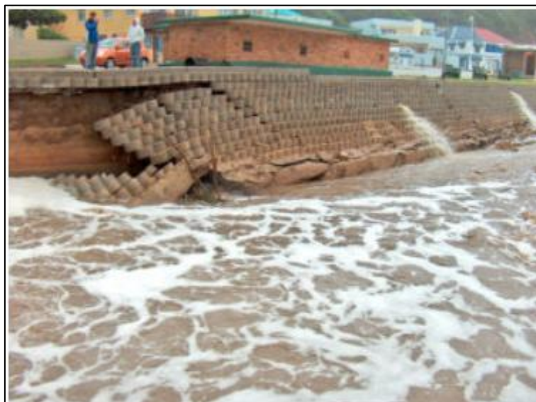
Figure 13: Failure of an interlocking concrete block wall at Herolds Bay in 2006 (terraforce.com, 2019)
