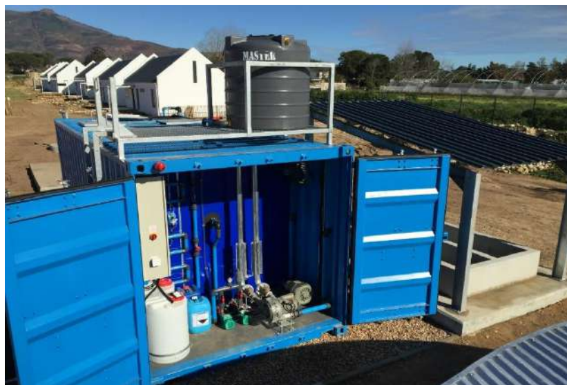
Figure 2: Image of a similar containerized package plant
