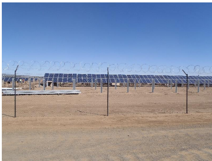
Figure A.8. Example of PV Technology (DEFF, 2019)
