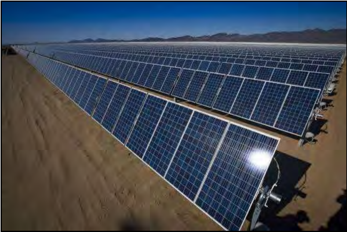
Figure 1.2: Typical PV SEF facility
