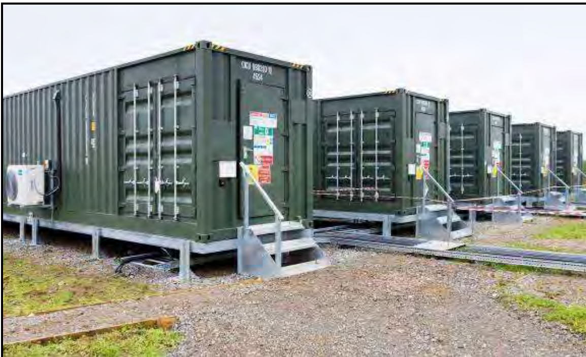
Figure 1.3: Example of BESS located in storage containers
