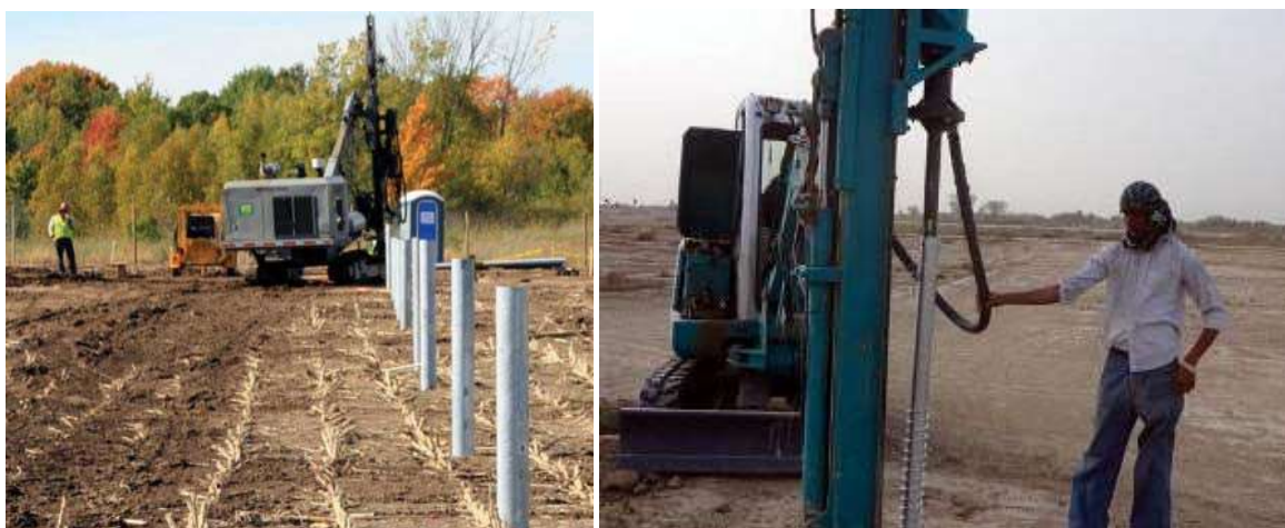
Figure 3: Driven/ Rammed Steel Pile (left) and Ground Screw (right) are the preferred mounting technology (Verbena PV, 2022)
