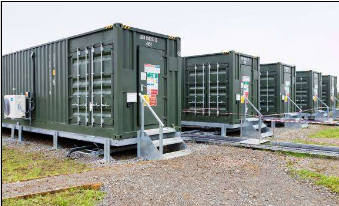
Figure 1.3: Example of BESS located in storage containers
